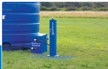
10,000 litre static storage connected to pump and tap stand.
