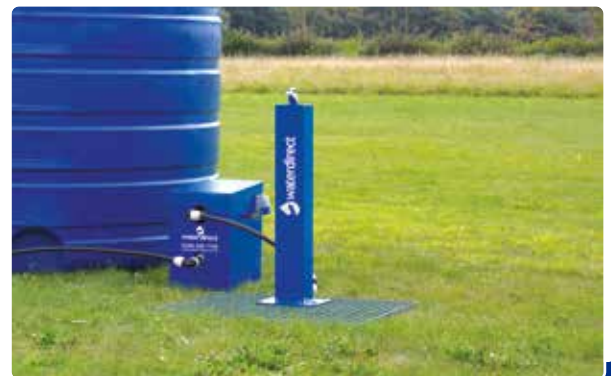
10,000 litre static storage connected to pump and tap stand.
