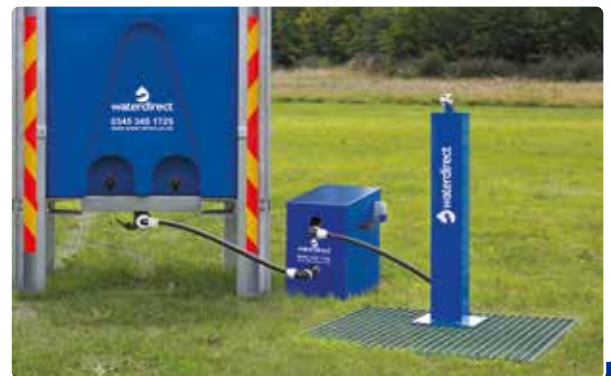
1,100 litre static storage connected to pump and tap stand.
